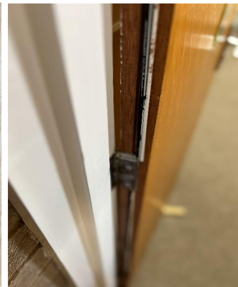
Damaged intumescent strips and cold smoke seals. Door opens onto a means of escape.
